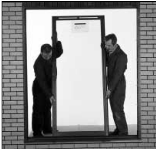
17 Lift the fixed door onto the plastic locating bar (bottom) utilising the temporary packer.
