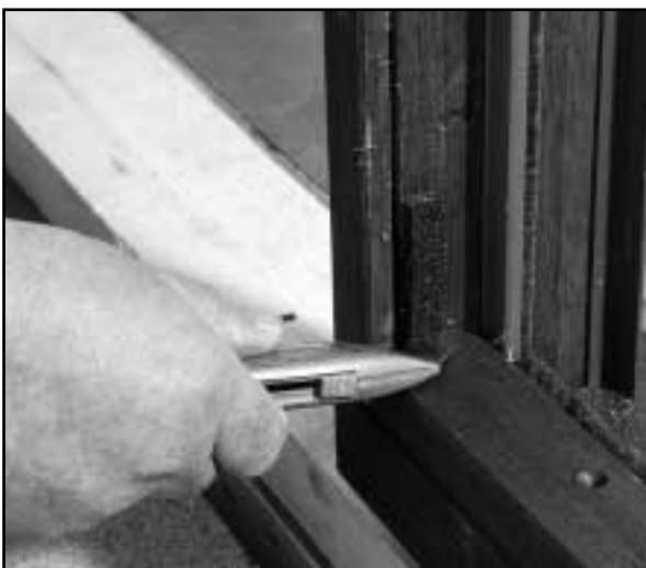
39 Trim the overhanging compressed tape flush to the top of the threshold.
